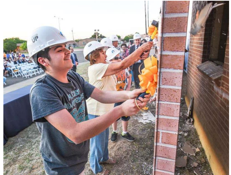
Residential construction begins at LHA's Russell Terrance, 2017 Photo Credits: Danny Zaragoza/Laredo Morning Times
